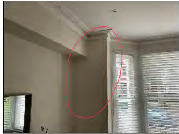
48 - Example of area where dampness was detected
