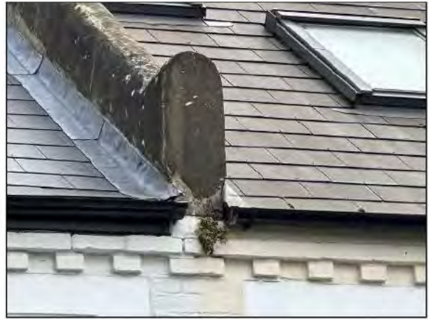
12 - Close up of vegetation and render damage
