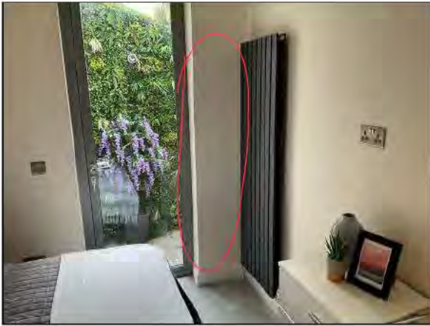
47 - Example of area where dampness was detected
