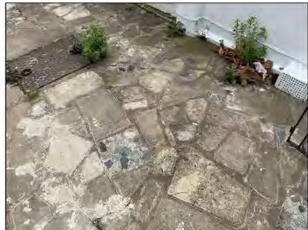
37 - Example of the damaged paving
