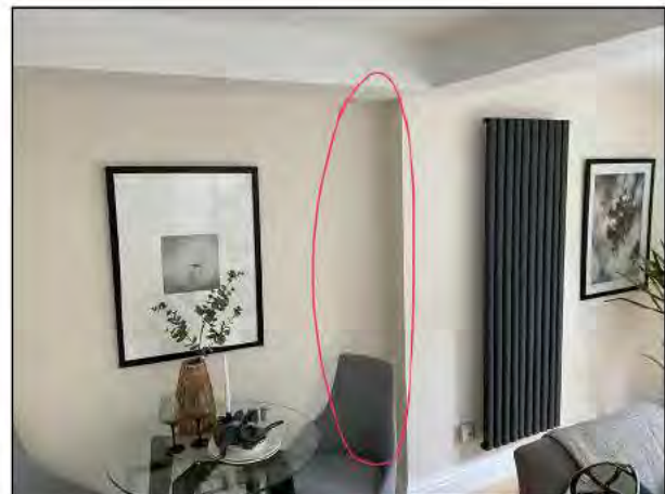
46 - Example of area where dampness was detected
