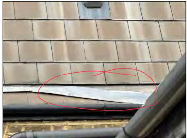
14 - Dormer flashing defective
