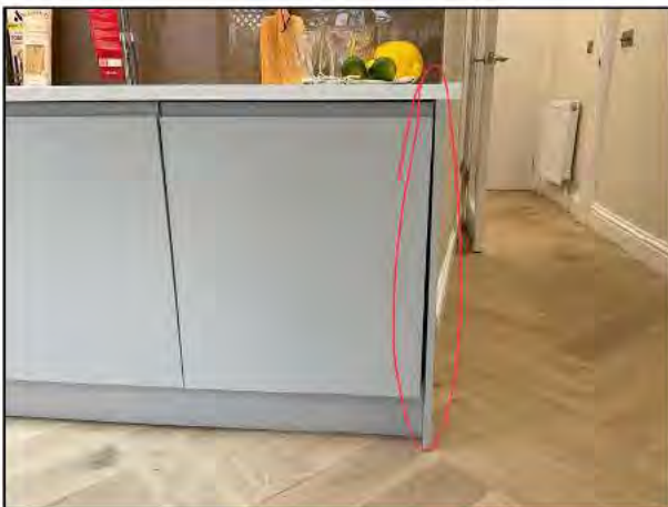
51 - End panel not level
