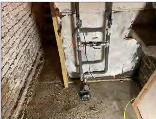
60 - Pump not connected
