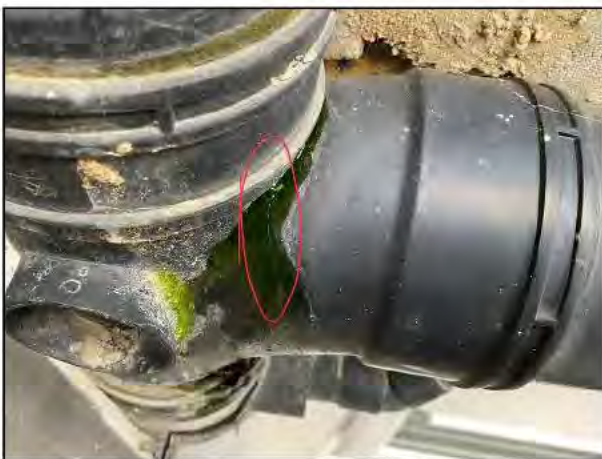
66 - Cracked soil pipe
