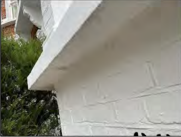
22 - No drip grooves
